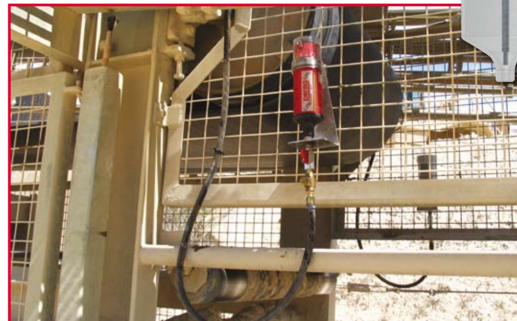
Remote mounted Perma Star Vario on conveyor pulley bearing.
