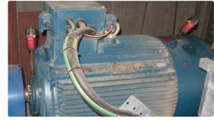
Electric motor bearings
